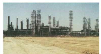
In 1966, the company won its first overseas business in the shape of an order for electrical equipment work in South Korea. It subsequently received orders in Pakistan, the Philippines, and Saudi Arabia, with its young and talented engineers making significant contributions to these countries. (Photo: Riyadh Refinery in Saudi Arabia)
