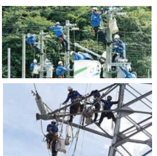
Distribution line education for new employees
