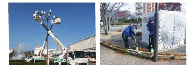
Cleaning streetlights in the Peace Memorial Park (Hiroshima City)
