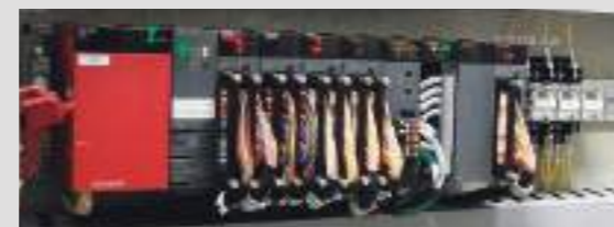
■ PLC(盤内) PLC (inside the panel)
